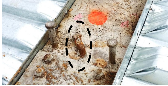
Figure 50 showing shear stud bend to a 90 degree angle as a result of being hit with a jackhammer during concrete removal. Shear stud is still attached firmly to the steel flange
